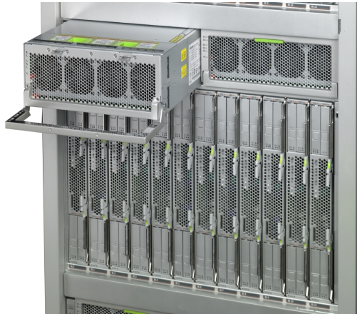
Power Supply Module Removed
